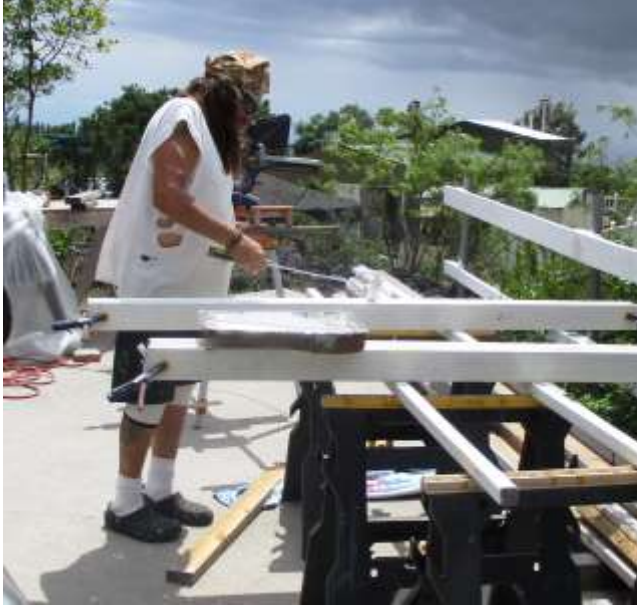
Steve Arguello puts the finishing touch on ramp handrail at McKinney Place.
